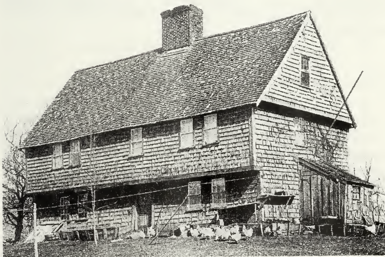
The Capen House in early 1880s. The lean-to shack served as a vestibule for the 18 th century west entry door. The arrow points to defective flashing and roofing at its junction to the gable wall were likely the cause of the extensive decay in the east girt still visible in the Hall.
